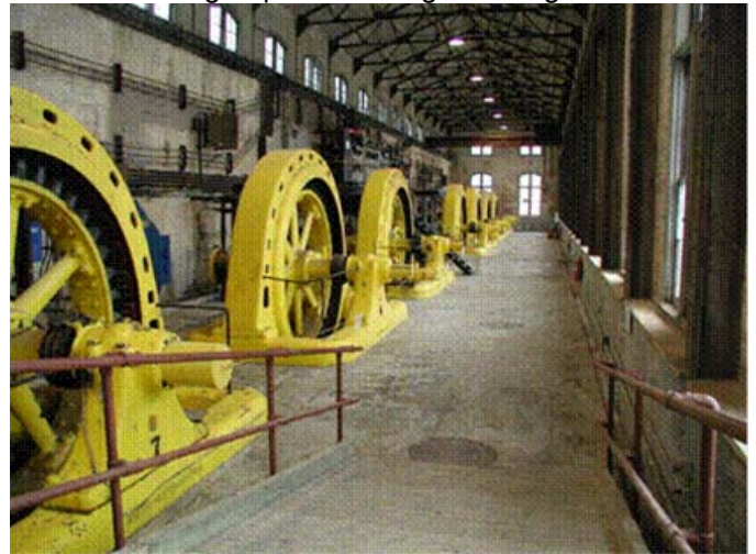
An inside view of the generating station showing the row of generators.
